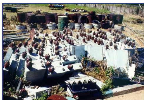
Temporary storage of transformers expecting elimination
