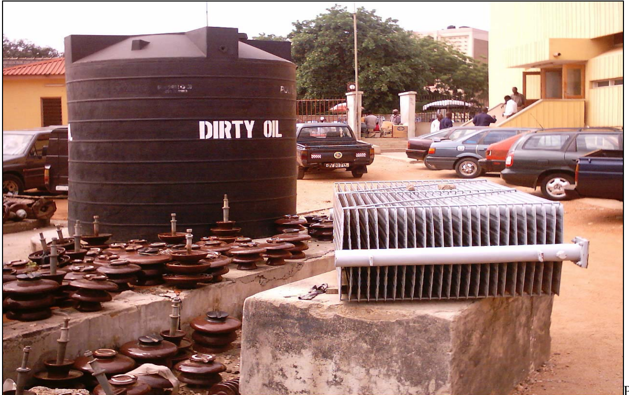
Plate 4: Displayed reservoir for PCB/oil waste at the Accra Central Power Station G
