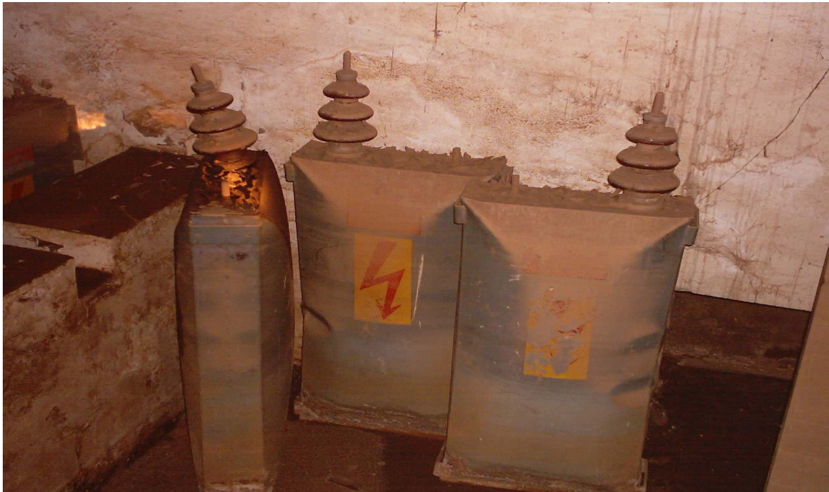
PLATE 6: CAPACITORS BROKEN AT THE INSULATOR END OR BULGING OUT ON THE SIDES
