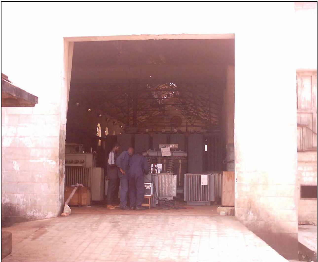
Plate 2: Technicians of the Electricity Company of Ghana at work in the transformer repair building
