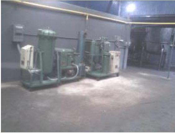
Pictures 5 and 6: Oil regeneration unit
