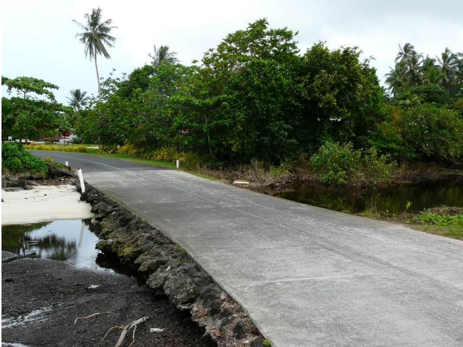
Photo 6: Road south of bridge showing water (on right) impounded by lack of culvert
