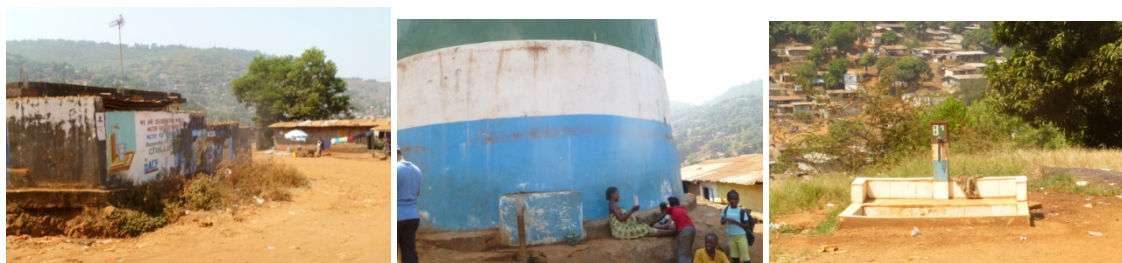
Figure 2: Images of the rehabilitated Mamba Ridge community reservoir, tapping the source of a local spring for water supply in an area of Freetown that does not benefit from supply from the existing Guma reservoir. The WASH consortium through Action contre la faim (ACF) has been implementing a community engagement project at this site in support of Guma Valley’s water supply efforts. The further development of alternative sources of potable water is seen to be an effective climate change resilience building activity.
