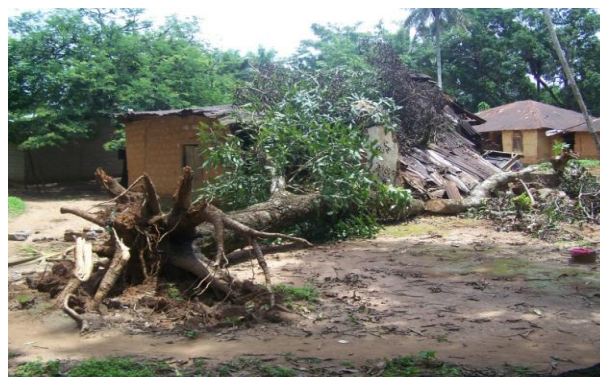
Figure 13 Result of flooding and strong winds in the Mambolo Chiefdom, Kambia District
