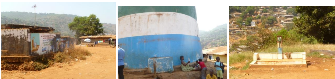
Figure 16: Images of the rehabilitated Mamba Ridge community reservoir, tapping the source of a local spring for water supply in an area of Freetown that does not benefit from supply from the existing Guma reservoir. The WASH consortium through Action contre la faim (ACF) has been implementing a community engagement project at this site in support of Guma Valley’s water supply efforts. The further development of alternative sources of potable water is seen to be an effective climate change resilience building activity.
