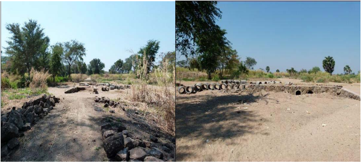
32. Figure 4: Destruction of infrastructure in Mangochi
