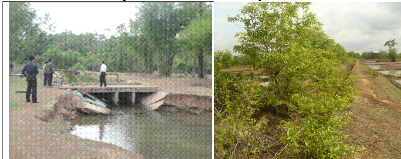
Picture 9: Culvert over an irrigation channel is unstable due to flash flood scouring the channel banks downstream from the culvert. The culvert foundation needs to be tied back and channel re-lined with concrete.
