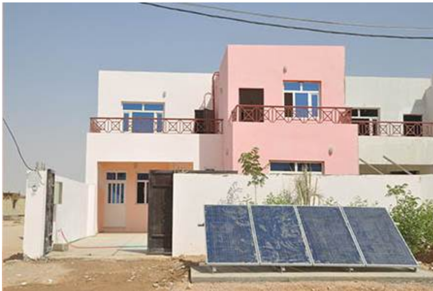
Figure 11. Test solar module installation at the Bytti Complex showing dust accumulation and effects of uneven cleaning.
