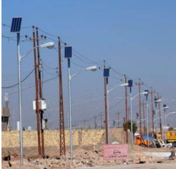
Figure 9. Solar street lights installed in Baghdad.
