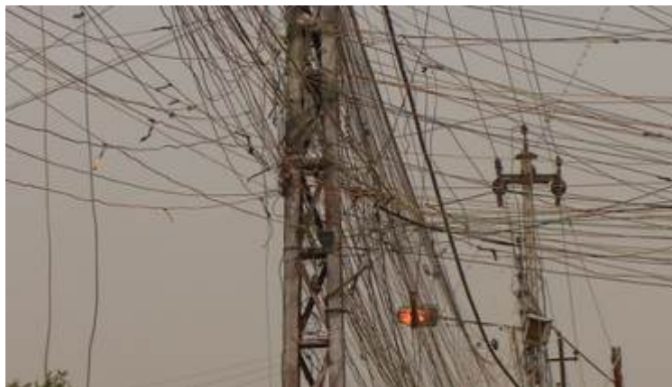
Figure 2. Ad-hoc power distribution grids established by entrepreneurs who run diesel generators to feed demand when the grid is down.
