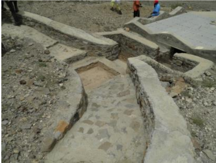
Figure 3: Canal system feeding into covered reservoir outside of Adailou
