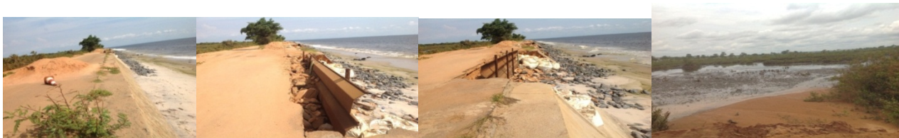
Figure 2. The effects of erosion on the Banana-Muanda road
