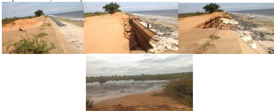
Figure 2. The effects of erosion on the Banana-Muanda road
