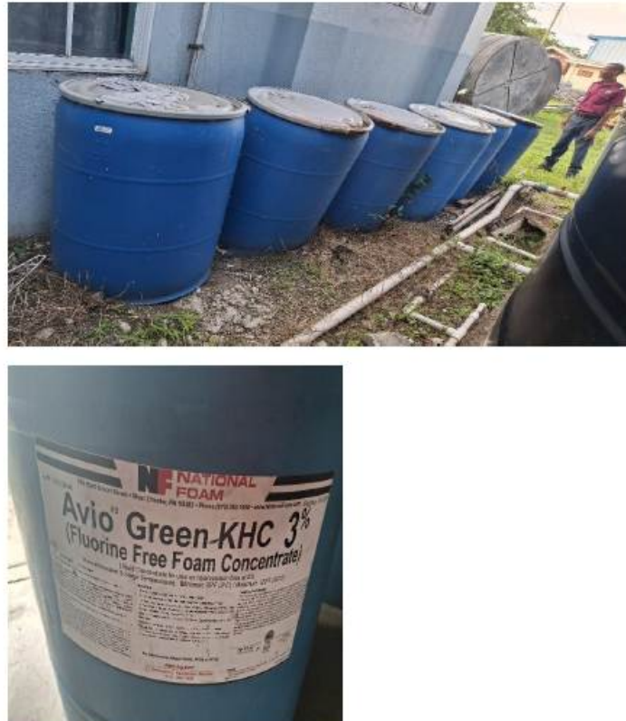
Figure 2. Foam Storage at the G.F.L. Charles Fire Hall
