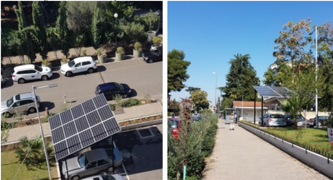
Figure 6: Recently built PV system in Tirana, used for road lighting and charging EVs, a business model requires wide-adoption and scale-up particularly in the southern part of Albania
