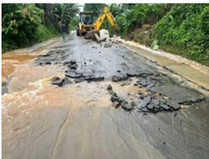
Figure 13. Floods in Principe destroy roads, 2022
