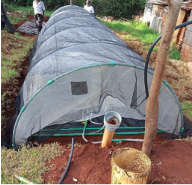
Prefabricated HDPE Flexi Biogas in Kenya
