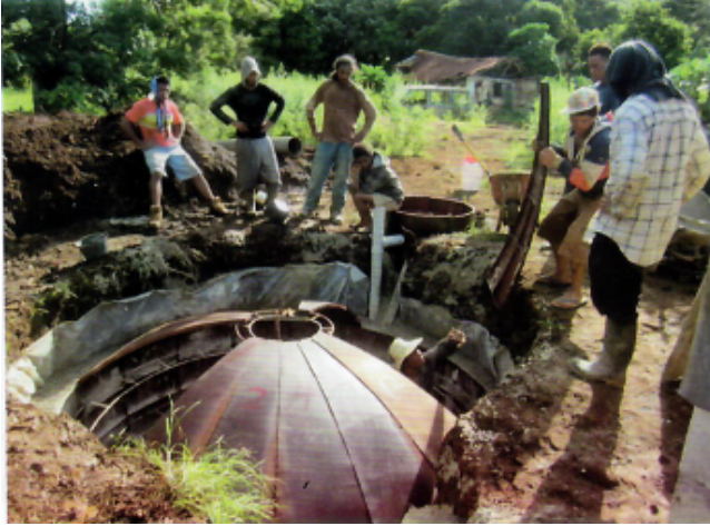
Fixed-dome Chinese model in Tonga (concrete using steel molds)
