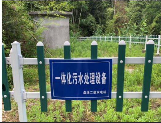
Sewage treatment facility in the Zhejiang Panxi Stage II SHP Station
