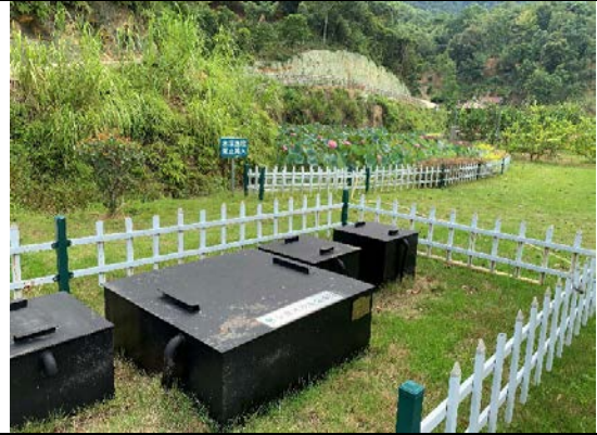
Sewage treatment system of Tangban Hydropower Station in Fujian Province
