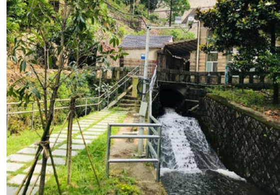
Ecological flow discharge facility in Panxi Cascade Hydropower Station in Zhejiang Province
