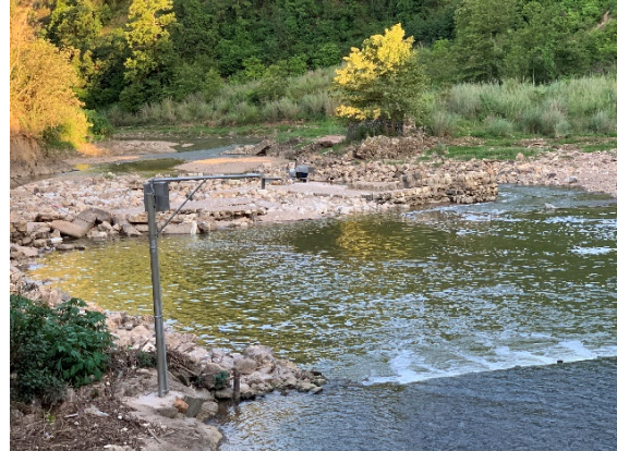
Online ecological flow monitoring equipment in Yunnan Mabozi SHP Station
