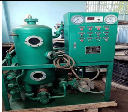
Oil filter in the plant of Chongqing Majing SHP Station
