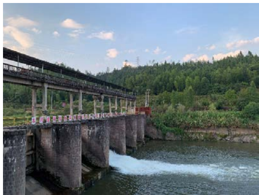
Discharge flow at Tantou Hydropower Station in Fujian Province
