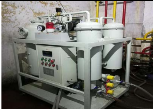
Oil filter in the power house of Guangdong Guanxi SHP Station
