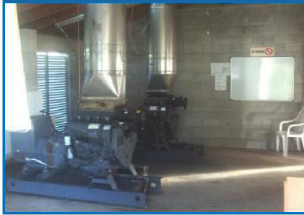
Photo 2: Existing Diesel Generators at Ha'afeva Power Plant
