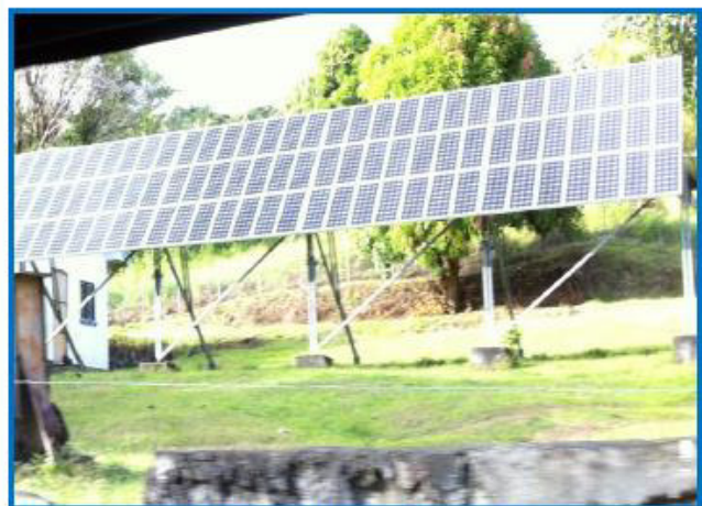
Image 2f: Solar Panels Installed for Telecommunication Centre in Niuafu'ou
