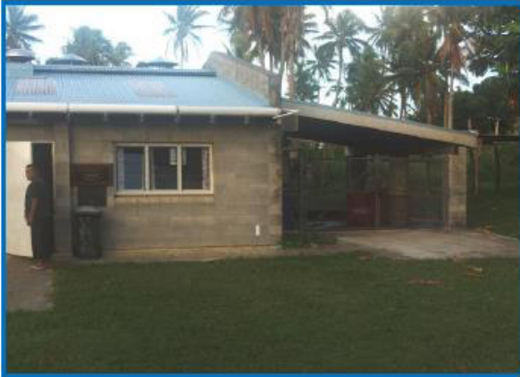
Photo 1: Existing Diesel Generation Station at Ha'afeva
