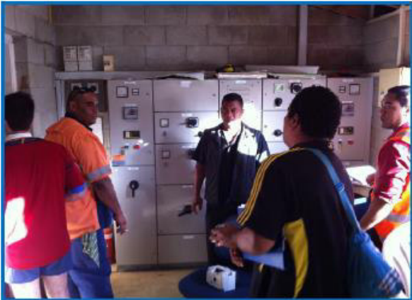
Photo 3: On-site discussion with Power Plant Technicians. Ha'afeva Island
