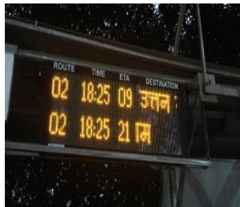
ITS - PIS display boards installed at bus stops in MBMC area
