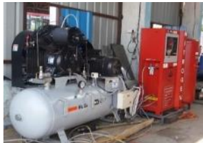
Air compressor installed at Depots
