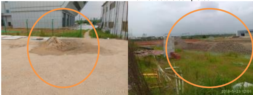
Construction material exposed without coverage
