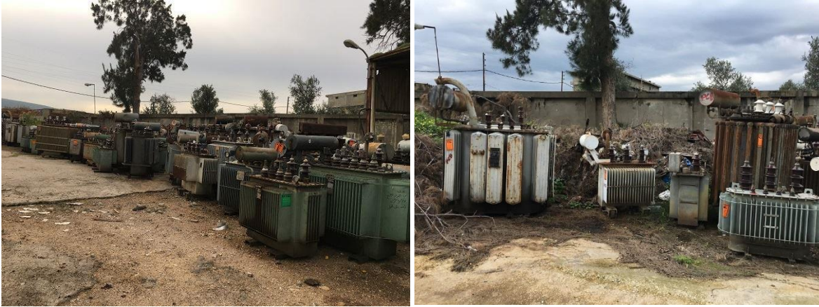
Figure C-4: Storage area for contaminated transformers
