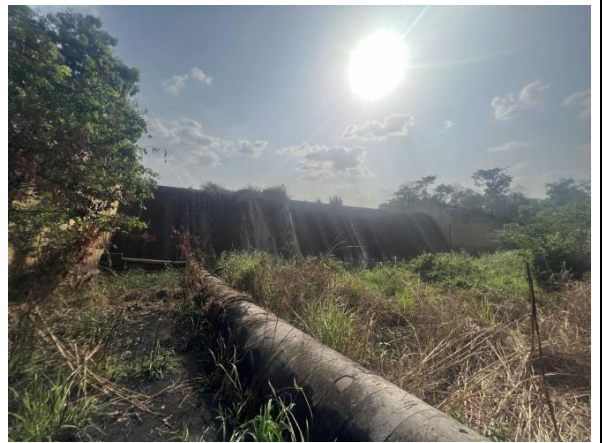
Figure 5-2.5 Penstock of the Proposed Hydropower Project of Itapaji Reservoir
