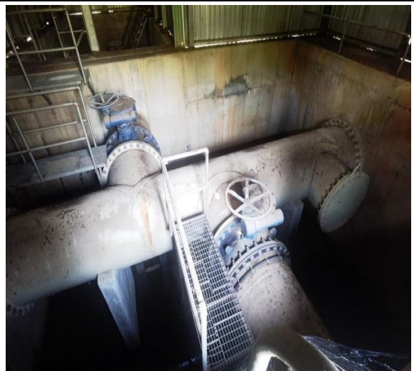
Figure 4-12 Water Transmission Valve Chamber of Owena Reservoir (Culvert Pipe Outlet)
