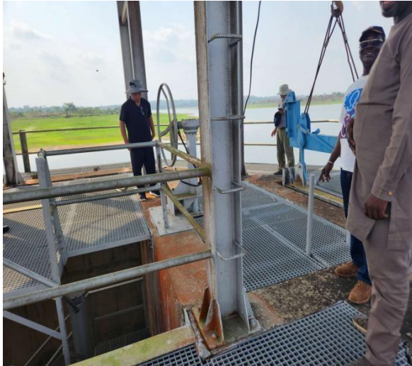
Figure 4-13 Water Transmission Gate of Owen Reservoir
