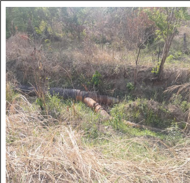
Figure 5-2.8 Bifurcated Penstock of Itapaji Reservoir
