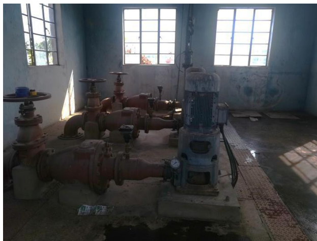
Figure 5-2.4 PS of Itapaji Reservoir (Urban Water Supply)
