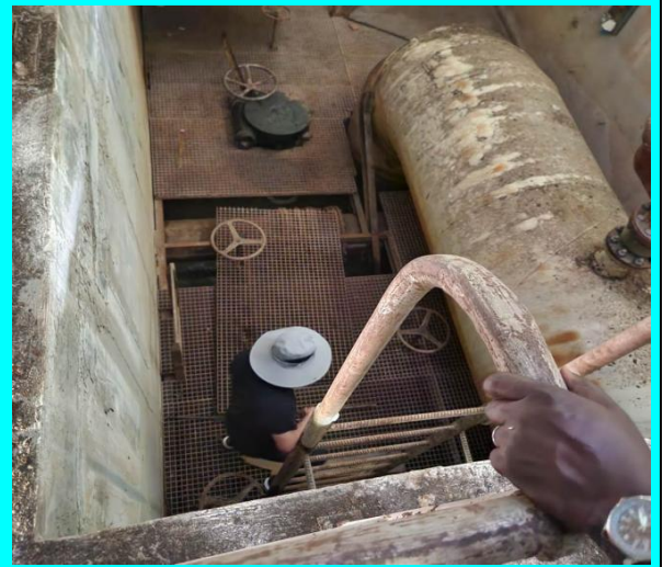
Figure 4-14 Valve Chamber at Outlet of Owena Reservoir
