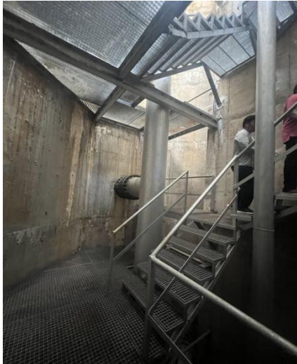
Figure 4-7 Inside the Water Transmission Gate of Owena Reservoir
