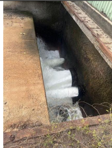
Figure 4-8 Water Release through Culvert Pipe in Owena Reservoir
