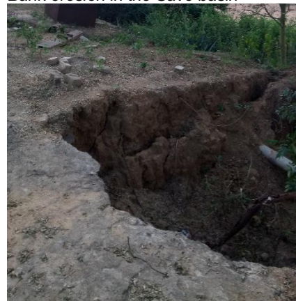
Bank erosion in the Save basin
