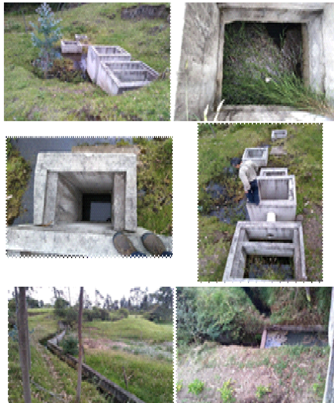
Figure 6. Wastewater treatment plant abandoned, municipality Montufar (Carchi province, Ecuador). The residual water contaminates the irrigation water.
